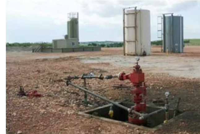
Waste injection wells (permitted)
