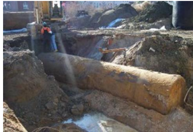
Underground storage tanks
