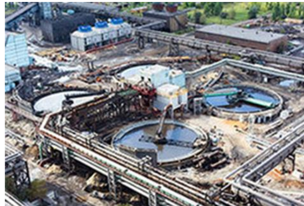
Leaking wastewater treatment
